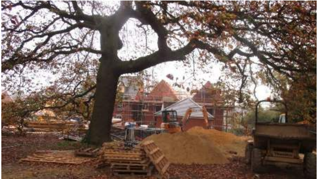
Figure 14. Bad practice: construction activities within the CEZ | DCC
